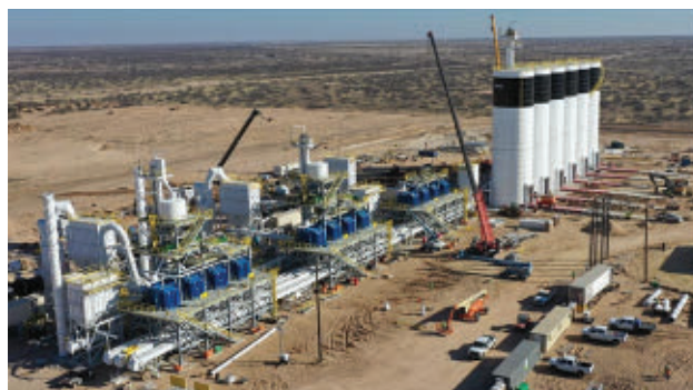
A dry sand plant is under construction in the Permian basin to reduce transport costs of sand. Massive driers on the left side of the photo dry the sand before it's tightly screened and loaded into the adjacent towers to be handled at the wellsite (Fig 4).
